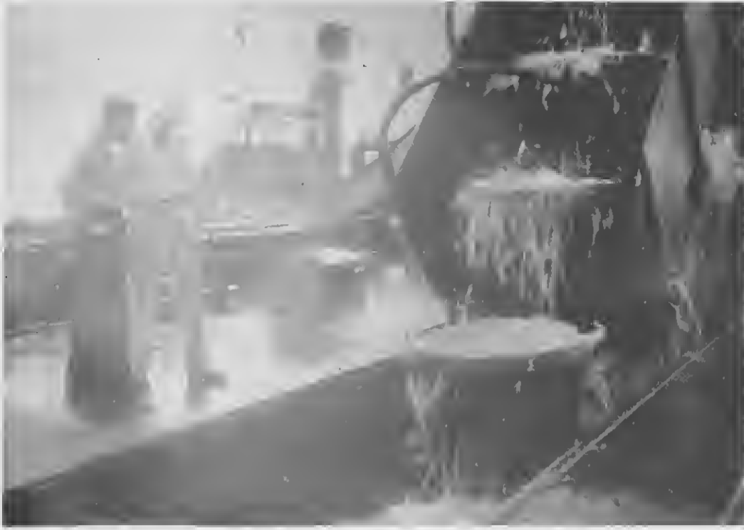
JAN VAN DER VLIES, dredge operator and Jan Hofman, superintendent of the San Nicolas Harbor project for the Royal Netherlands Harbor Works Co., watch the spoiling buckets come up from the bottom.
